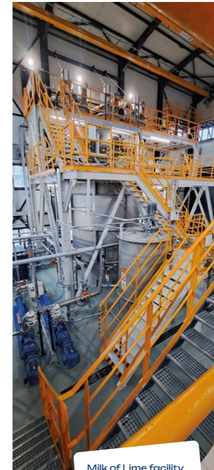
Milk of Lime facility
